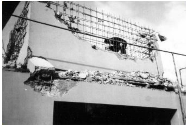
Figure IX: Damage to a more modern building from the 1974 earthquake in Lima, Peru (LimaEasy)
